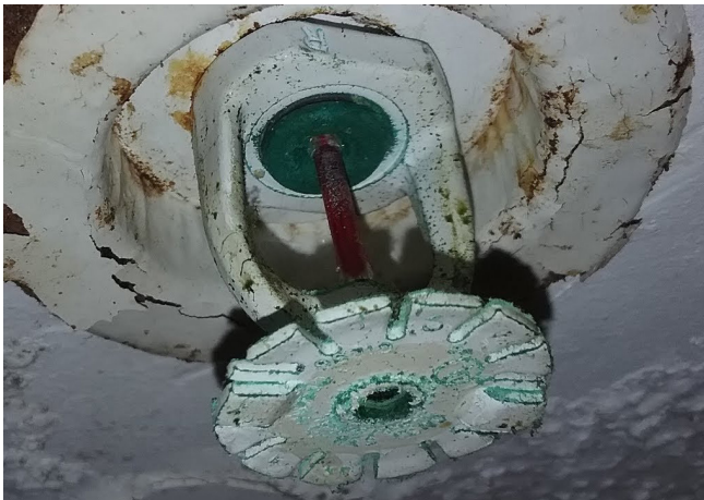
A Corroded Sprinkler Head
