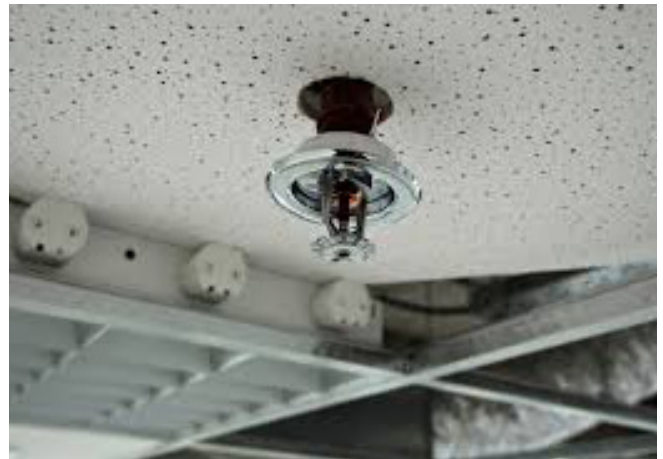
B Loose Sprinkler Hardware
