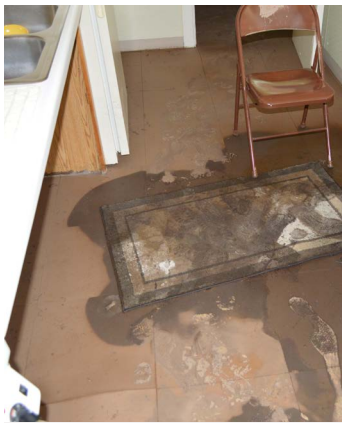
Arapahoe Court units sustained heavy flood damage.
