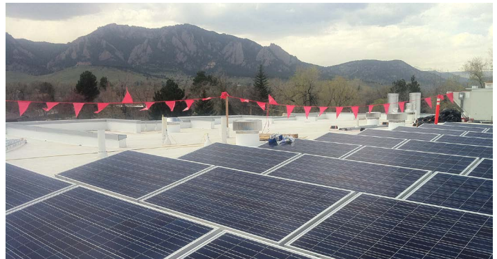
A 130Kw solar array is installed on the roof and carports at High Mar, BHP's newest completed development project.
